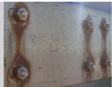
Bimetallic corrosion of mild steel bolts coupled with stainless steel plate.
