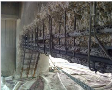
Pitting of mild steel reinforcing bars in a marine environment.
