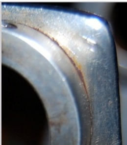
Crevice corrosion at the perimeter of a flange fitting.
