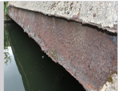
Uniform corrosion on a carbon steel beam section.
